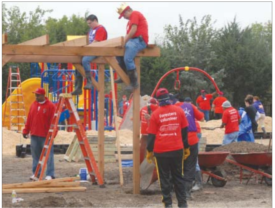
Working for the fun of it, volunteers steadily make progress while building a new playground for the Universal Academy's Irving campus.
